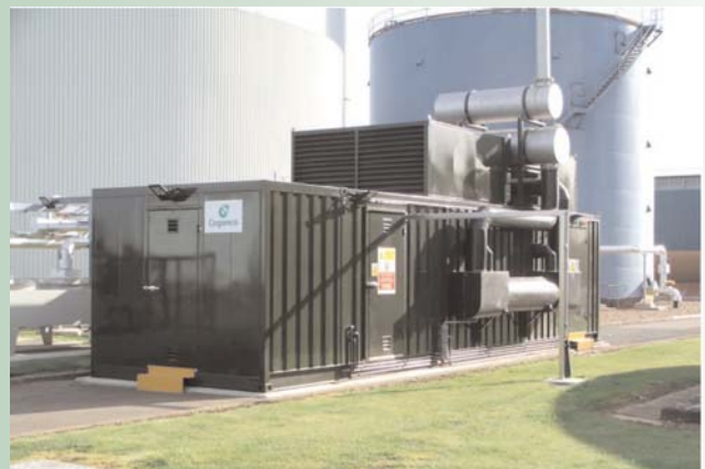
COGENCO 300 kWe unit in Cambridge, UK
