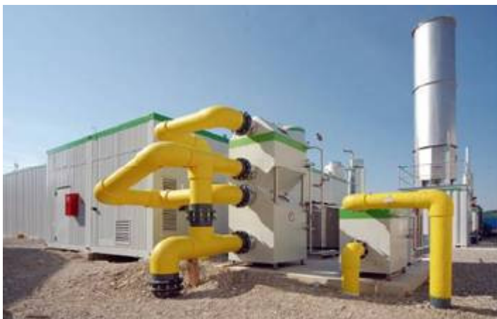
Gas feed-in Plant Pliening (near Munich)
